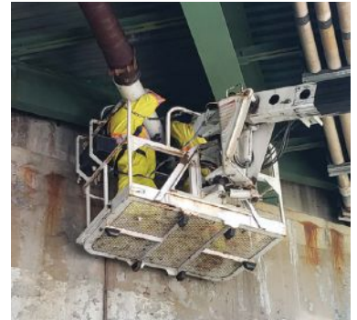
PPM crew is installing SRS sleeve and PVC pipe between abutment wall and gas main
