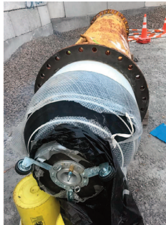
The inflatable "bladder" designed to inflate inside the pipe segment, ensuring that the adhesive liner was flush with the pipe
