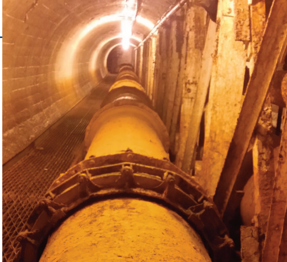
Tunnel underneath Gowanus dates back to the 1880s. Note the detailed brickwork on the walls.
